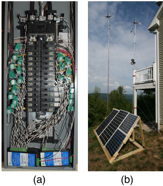
Figure 1: CT installation at the mains panel in Home A (a); solar panel and micro wind turbines at Home C (b).
